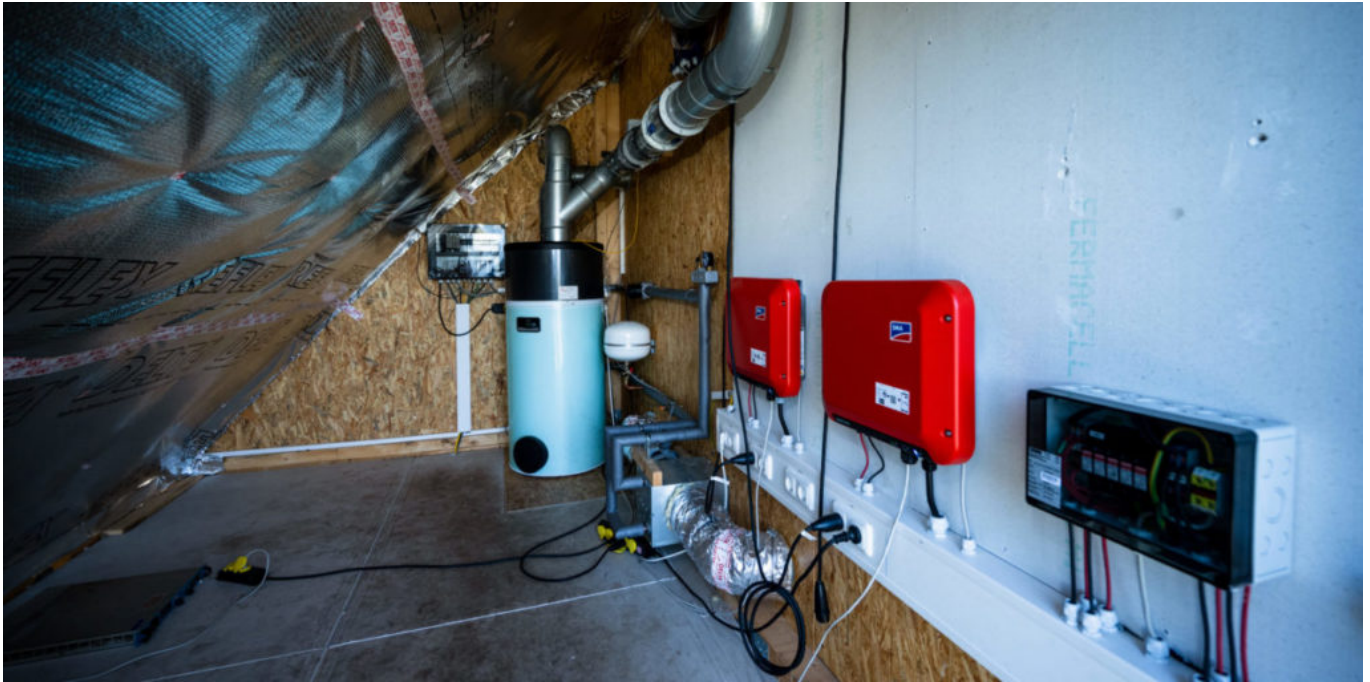
The solar system preheats air for the coupled air heat pump. Image: Costa Belibasakis/TH Köln
